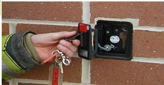
Knox Box Inspection & Key Verification
