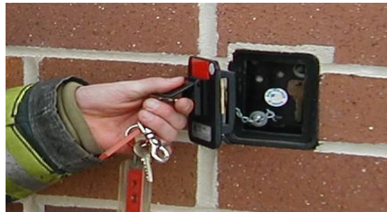
Knox Box Inspection & Key Verification
